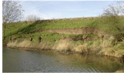
riverward macro- instability
